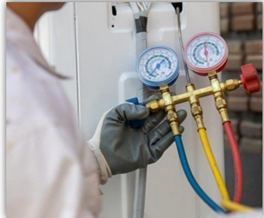
Image: Refrigerant charge verification testing
